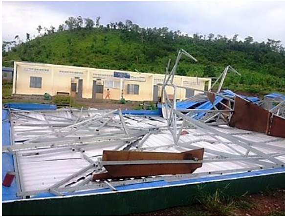
(Tin roof destroyed by Typhon)
