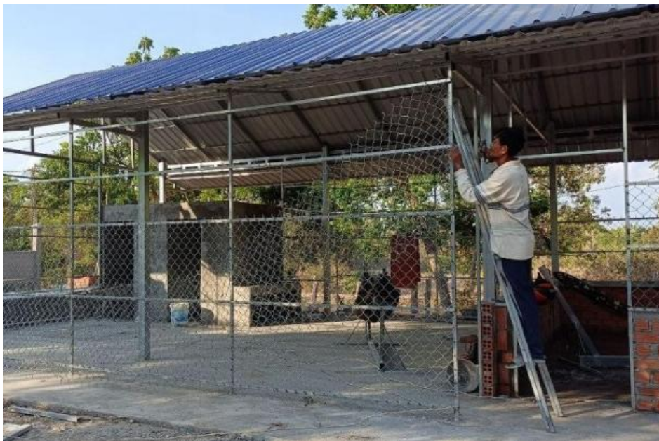
From day to day, the building was progressed, Dr. Samnang as project the responsible person for this construction was usually keeping monitoring to see the construction progress including quality of material for building (Dr. Samnang and his field supervisor visiting the progress of construction)
